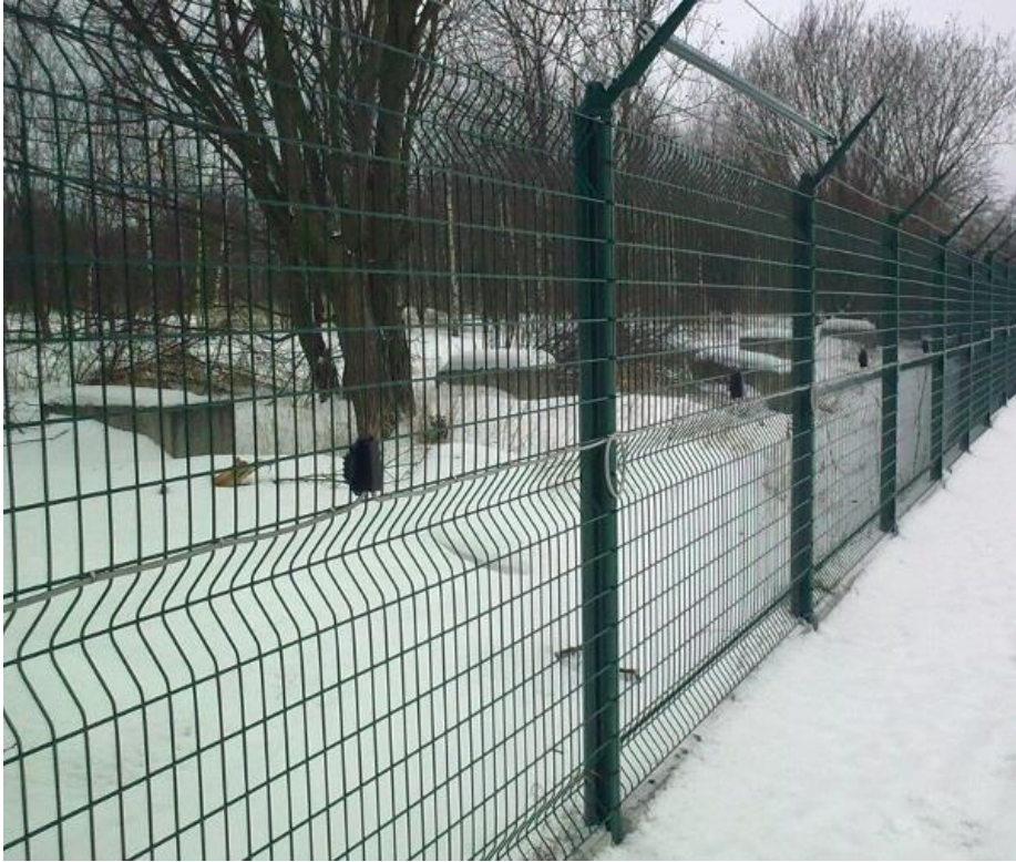
Detector placement and the method of running the cables across the fence
