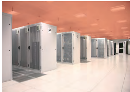
Ceiling protection at Data center
